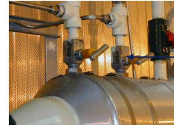
Needle valve installed providing 1/8" hole in sensing X
