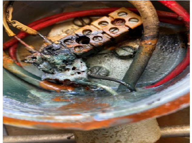
Figure 3: Severe corrosion on wiring terminal between indication switch and RTU causing activation indication.
