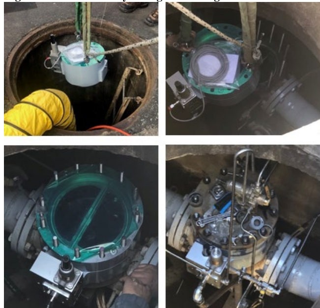
Figure 1: 6-inch Mooney Flowgrid below-grade retrofit.
