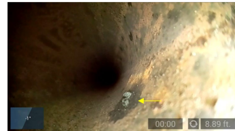
Regulator No. 1 through Regulator No. 2 Loose debris
